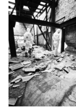
Big storage room with destroyed roof where samples No. 10, 24 and 17 were taken.
