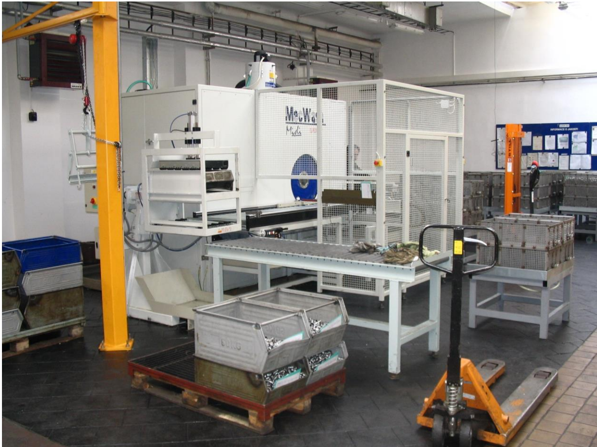
Figure 6: New Midi 400 degreasing equipment in the Brisk Tábor facility. Thanks to its installation, the spark plug manufacturer was able to replace tetrachloroethylene, used in the manufacturing process before. The equipment was installed within the framework of the environmental project “Degreasing of metal parts” supported by the State Environmental Fund. Photo: Brisk Tábor, a.s.
