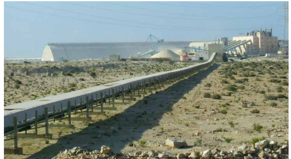
Photo 4.11: The final segment of the 98 km-long conveyor belt, transporting phosphates to the Port of Laâyoune. Photo by Pera Outdoor via Panoramio on Google Earth.
