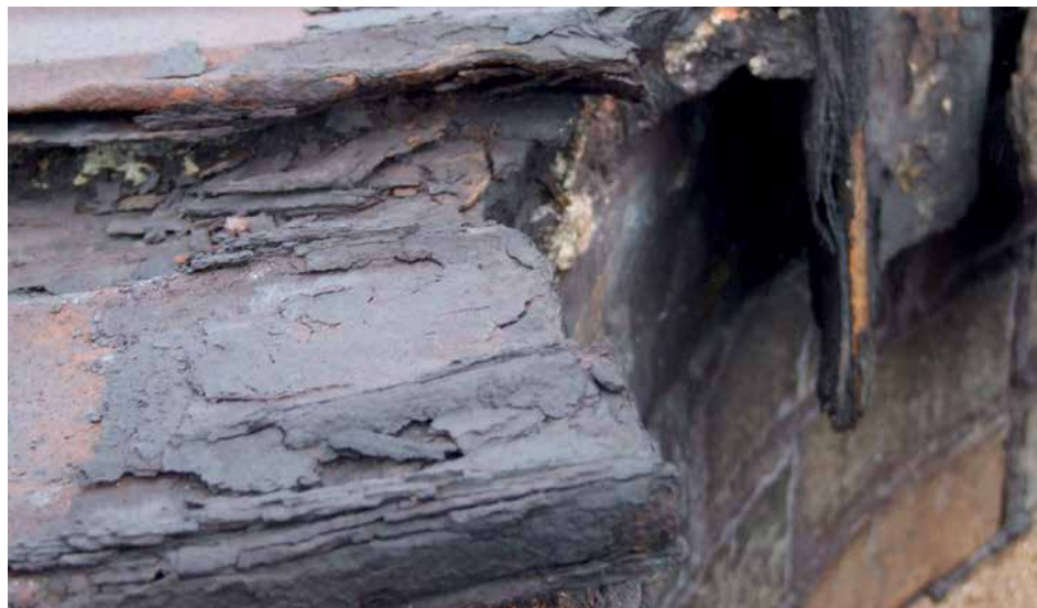
Photo 9.4: Corroded iron lining of a decommissioned waste incinerator chimney. Photo: Arnika's archive.
