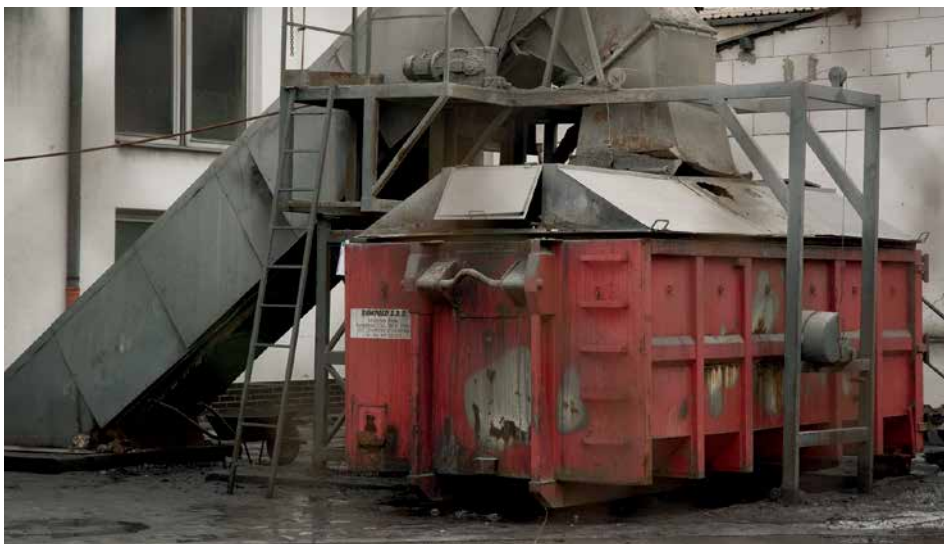
Photo 4.6: Fly ash from incinerators is a major source of dioxins and escapes control due to lenient limits. Equipment for collecting and transporting fly ash from hazardous waste incinerator in Jihlava, as it looked in 2012. Photo: Matěj Man, Arnika.
