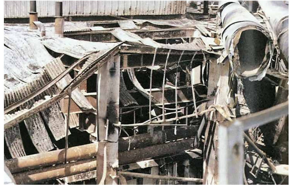
Photo 7.2: What remained of the original incinerator in Vienna – Spittelau after the fire in 1987. (Source: Wien Energie, 2024).
