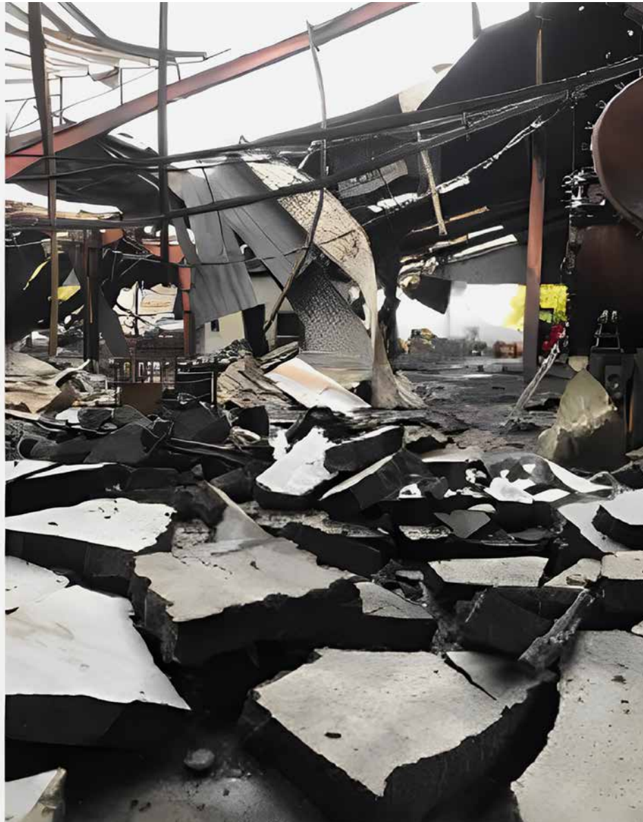
Photo 7.18: Walls toppled due to explosion, roof gone (2021). (Source: Hedlund, 2023).
