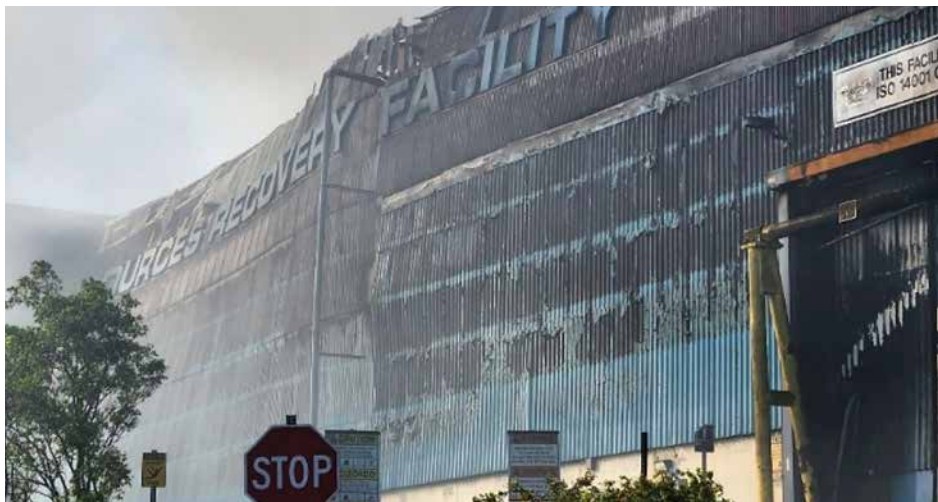
Photo 7.23: Exterior of the Miami-Dade County Resources Recovery Facility after a fire in February of 2023. (Source: Burkhardt et al., 2023). Photo: Miami-Dade County Department of Environmental Resources Management
