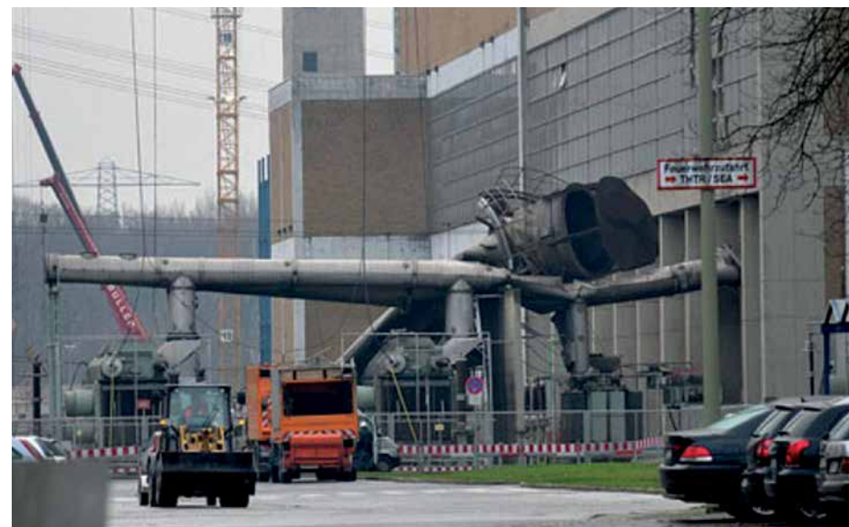
Photo 7.16 The Hamm pyrolysis stack corroded and collapsed in 2009. It was never rebuilt. Photo: Reiner Mors, tz.de, Source (dpa, 2009).
